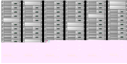
Fig. 1. A row of racks in a data center
