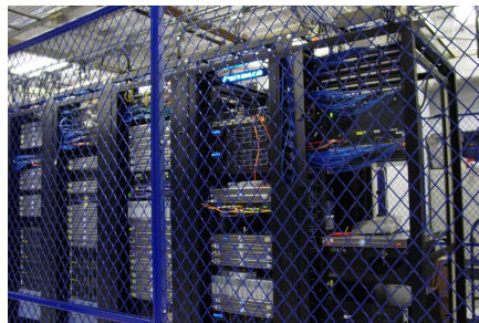
Fig 1. Snapshot of row in a data center
