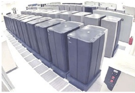
Fig 1: Physical organization of a data center
